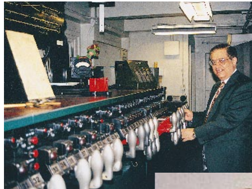
NYCT's Dr. Nabil Ghaly at the controls of a 60-year old mechanical interlocking still used today to control trains.
