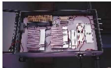
Kasten Chase's RF Routers are housed in a NEMA enclosure along the wayside. Also in the enclosure are a power supply, a combiner/splitter and two fusion splicing trays for optical fibers.
